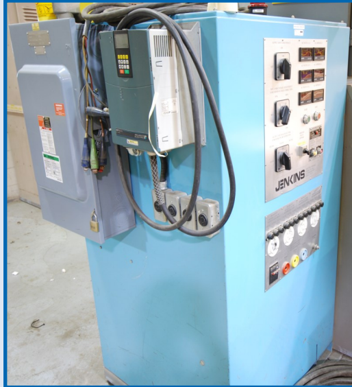
JENKINS ELECTRICAL TEST UNIT
